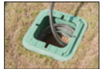
Slack Cable Storage in Small Base
